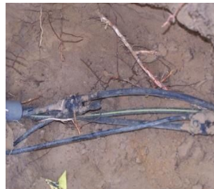
Pre-Meter Power Theft
